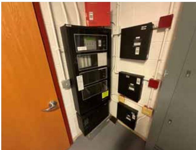
29 - FIRE ALARM SYSTEM
